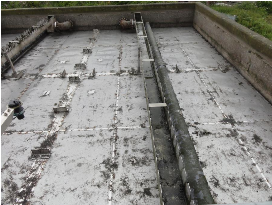
Image of an empty tank (SWW Plympton plant, June 2017), showing the position of the steel mesh screen in the reactors.
